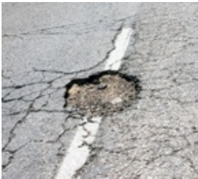
Figure 10: Typical small pothole with missing pavement.
