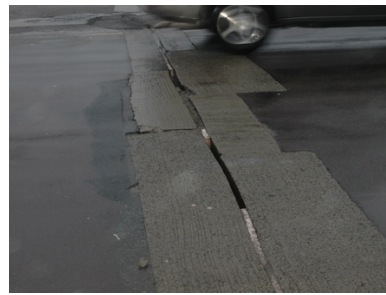
Figure 12: Borderline expansion joint, on a high-speed bridge. This generated a pothole detection.
