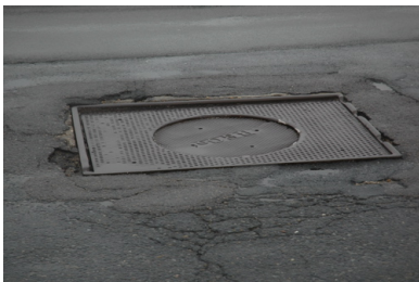
Figure 11: Severely sunk-in manhole, with eroded edges. This generated a pothole detection.
